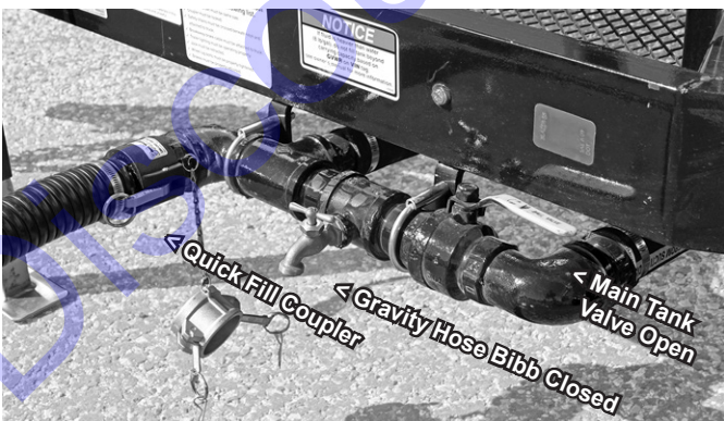
Figure B4 Filling Tank From Pressurized Source
