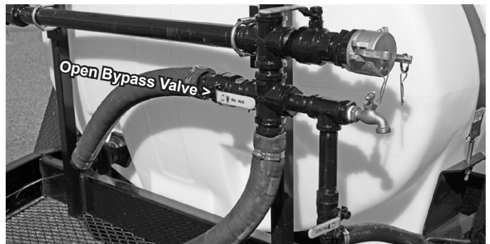
Figure B6 Open Bypass Valve
