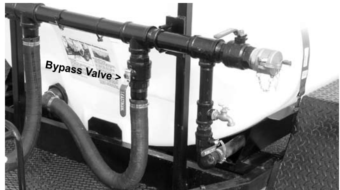
Figure B6 Open Bypass Valve
